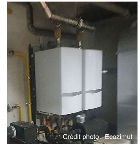
Chaudières VAILLANT ECOTEC + 1006/5-5
